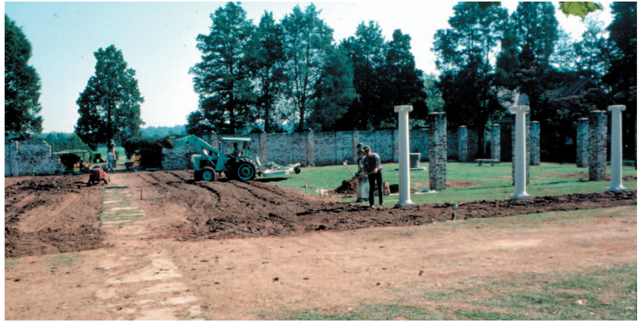
Fig. JJ: Garden restoration showing gate reconstruction and soil removal to expose bed layout. (Reed Engle)
